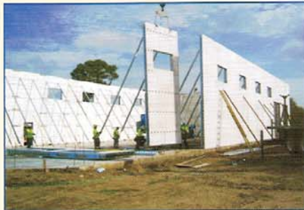
After the forms are positioned they are filled with concrete on site, creating a single continuous structure.
